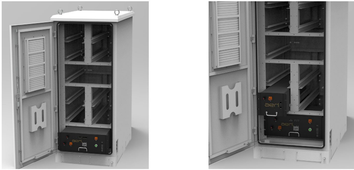
FIGURE 5.3 The BMS goes in first, at the bottom of the string.
